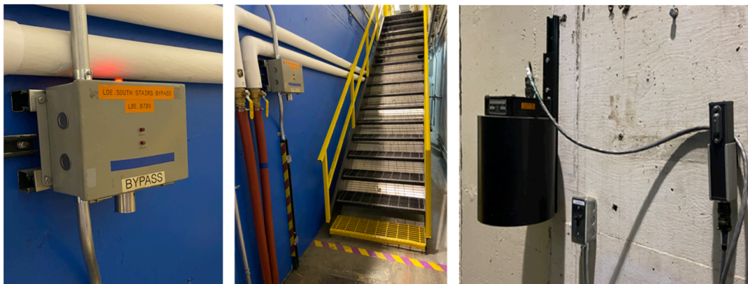
Figure 2.8-26: Personnel protection system hardware – bypass (left), light beam and bypass at stairs to mezzanine (center), and radiation monitors (right).
